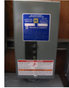
Example: Single slot 70A breaker box with 40A breaker
