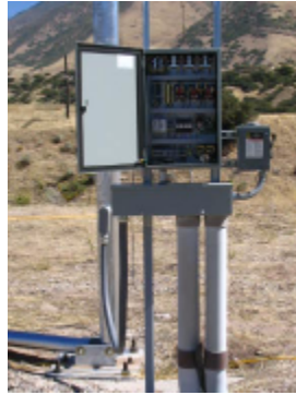
Example: Tower control panel tied (with nipple) to gutter box. Tower base lockable disconnect shown on far right
